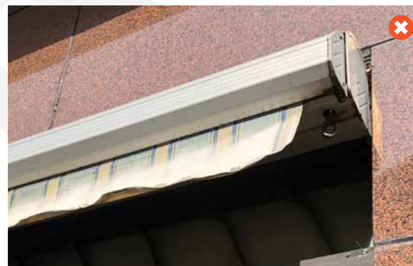
Figure 47. Blind box not well integrated with shopfront
